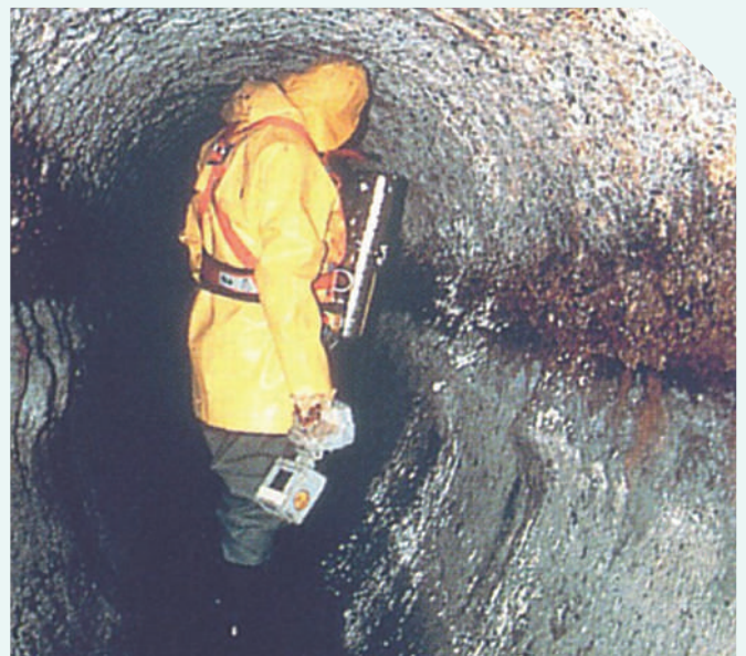
Figure 2: Sewer with BSAC
