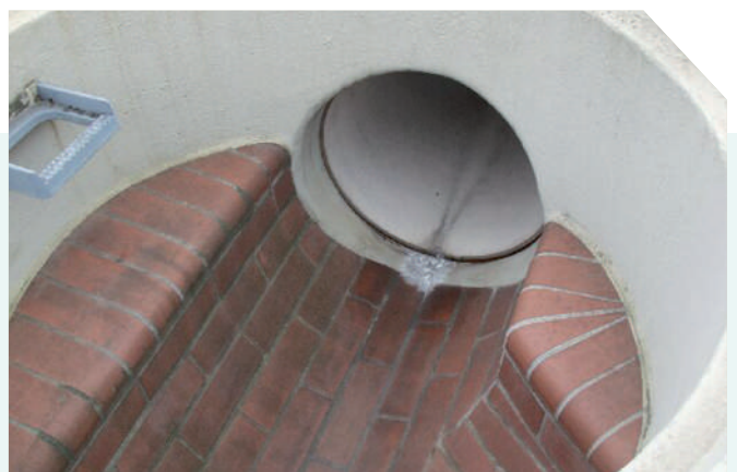
Figure 8: Sewer access shaft made of ISTRACA 50
