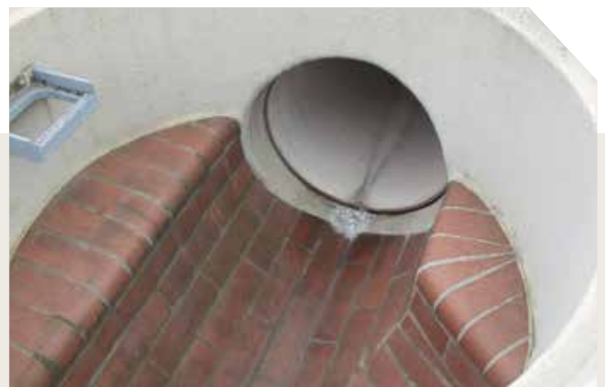
Figure 8: Sewer access shaft made of Istra 50
