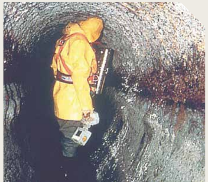
Figure 2: Sewer with BSAC
